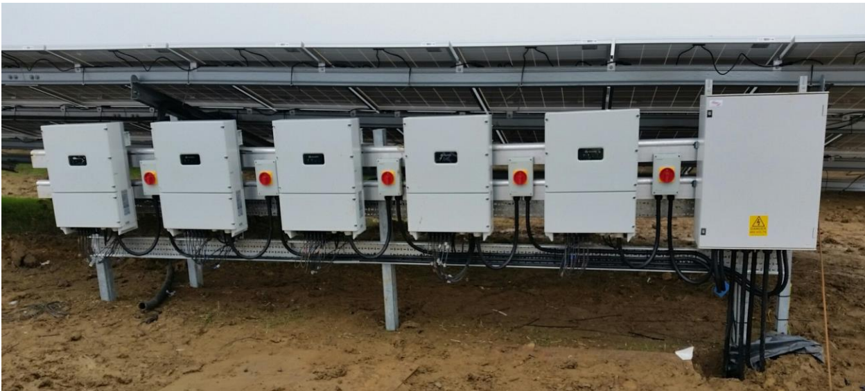
Plate 2-3: Typical string inverter installed under PV modules
