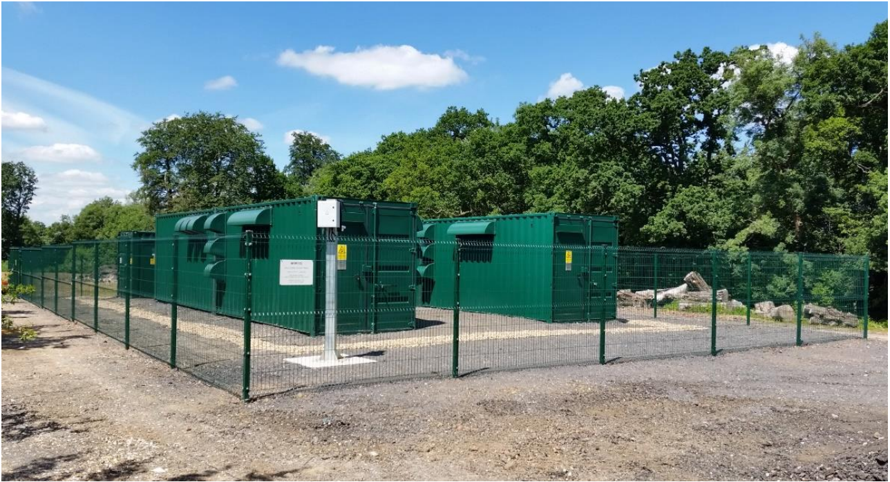
Plate 2-4: Typical central inverter
