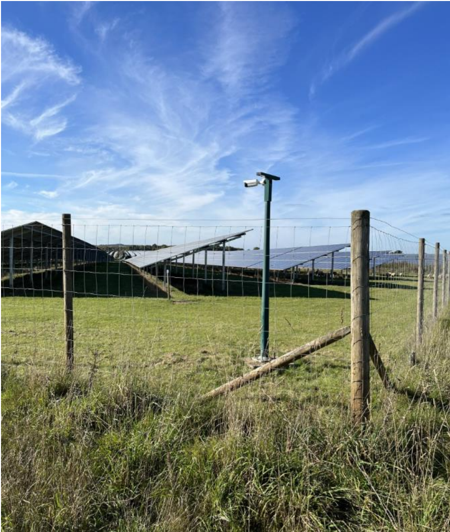
Plate 2-7: Metal CCTV pole and 'deer fence'
